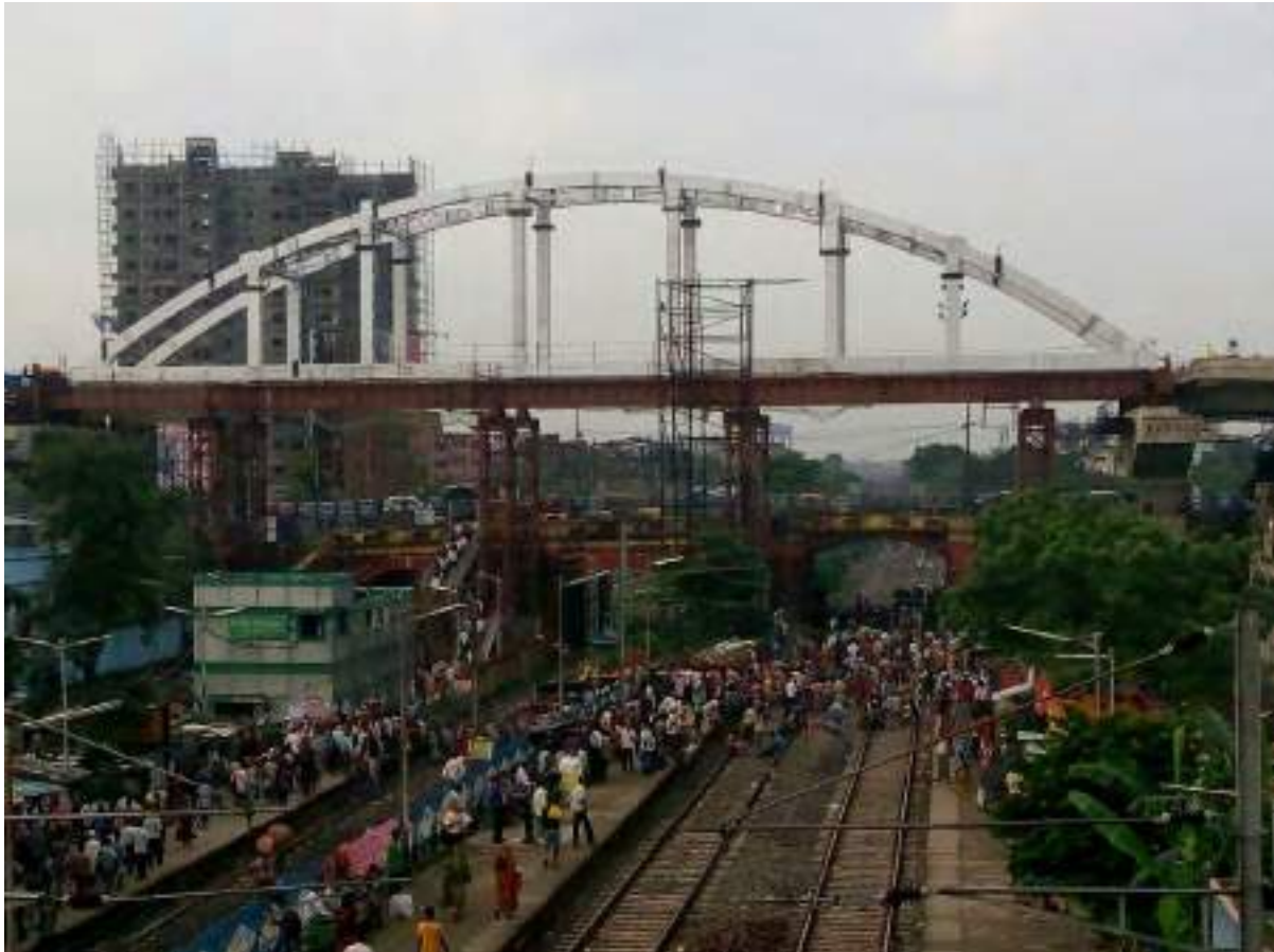
Fig 2 Photo: View of Bow String Arch Girder from Railway Station during construction stage (Park Circus station of Eastern Railway)
