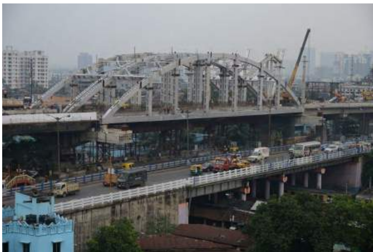
Fig 1 Photo: View of Bow String Arch Girder during construction stage (Park Circus station of Eastern Railway)
